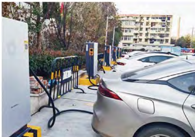
Guozhen Plaza EV charging station in Hefei, China
