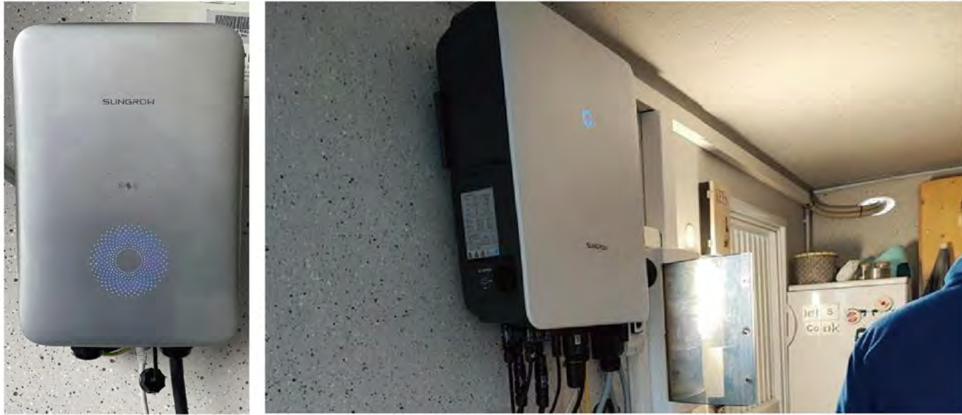
Residential PV+ESS+Charger station, Germany 🇩🇪
