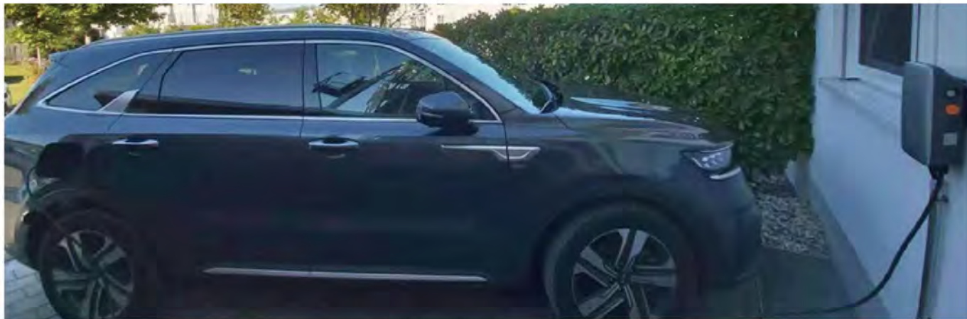
Residential PV+ESS+Charger station, Germany 🇩🇪
